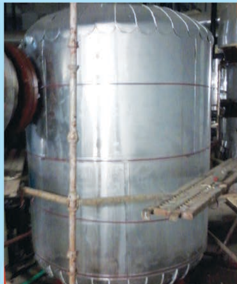
Chilled Water Tank
